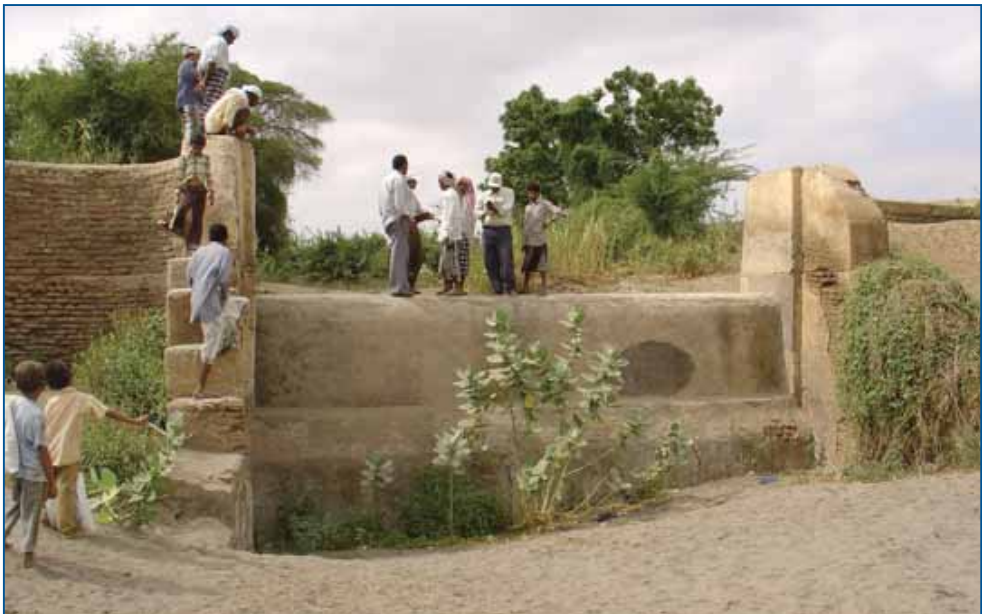
FIGURE 4.21 Stepped drop structure, Wadi Zabid, Yemen
